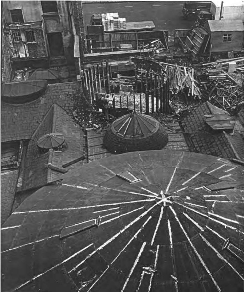
Figure 9.3a Demolition of the Rotunda site in January 1958. The circular roof of the small theatre of the Rotunda.
