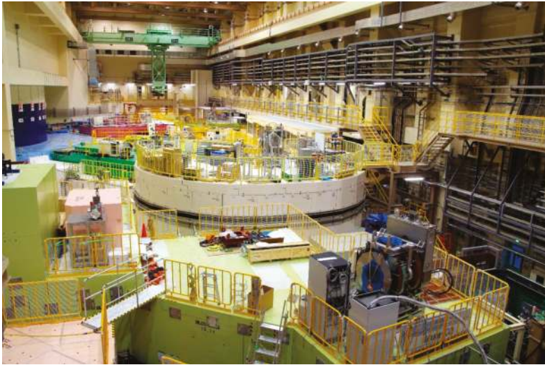
Figure 3. Photograph of the Materials and Life Science Experimental Facility (MLF) Experimental Hall II at J-PARC with the muon D-line shielding in the foreground and looking over the neutron beamlines BL14 in the image center to BL23 at the far back (compare to Figure 2).
