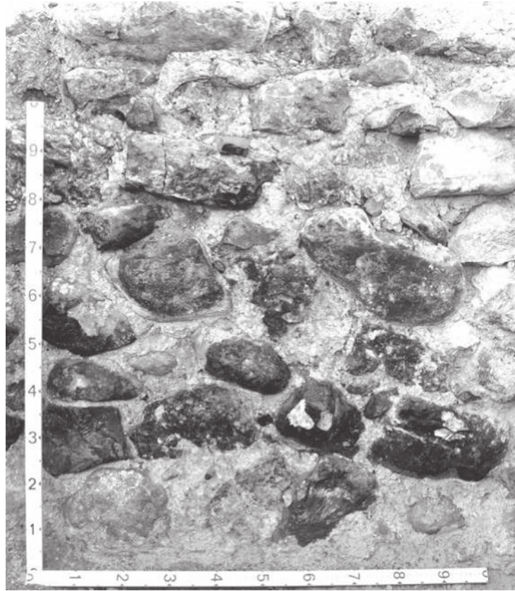
Fig. 252 Soot on northern wall of Room 19
