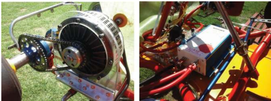
Figure 8. PMDC 10 kW motor and Q1 450 A controller.
