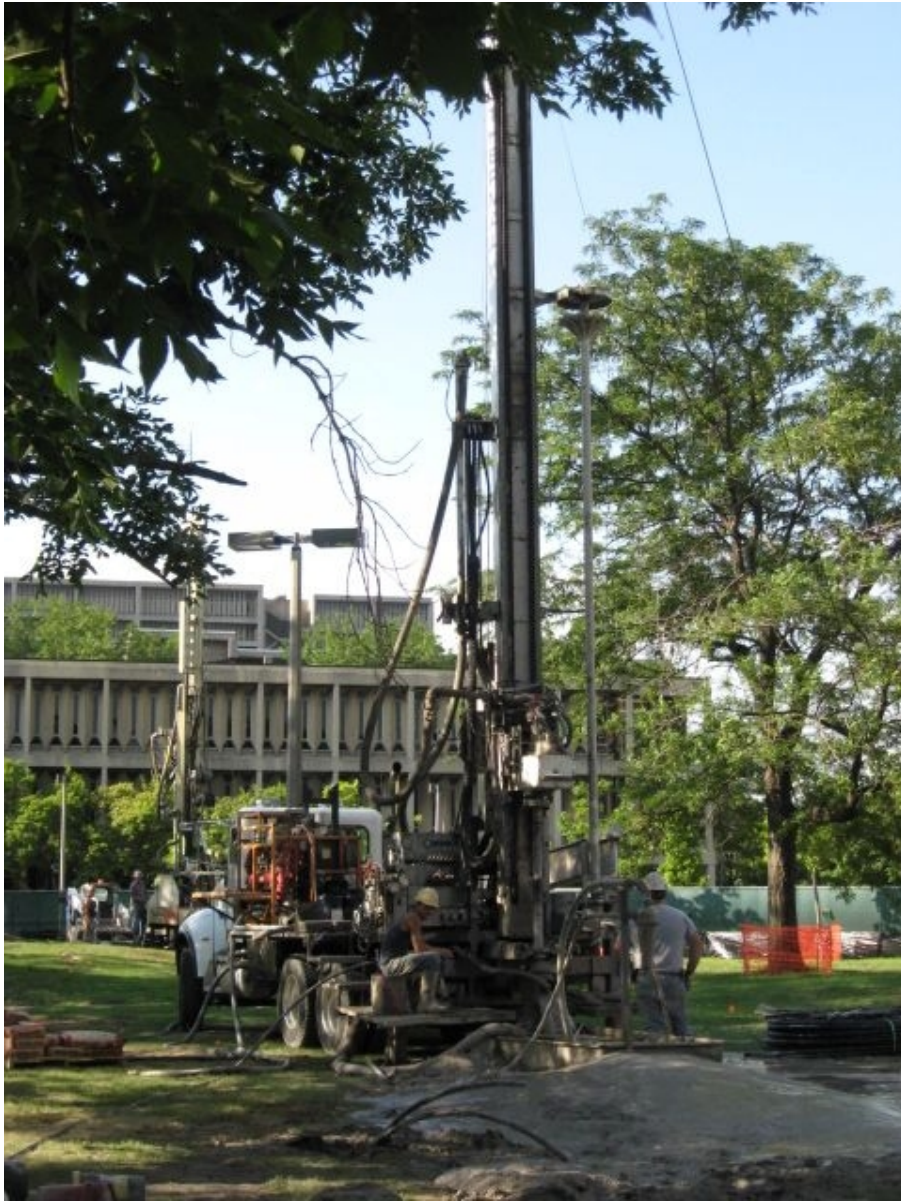
Figure 8.16: Installing a Geothermal Pipe System Drilling to install geothermal ground source pipe system. Source: Office of Sustainability, UIC 45
