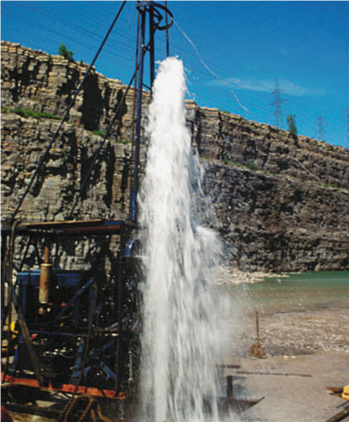
Figure 5.14: A Flowing Well Flowing artesian well where water moves above the land surface due to extra pressure on the groundwater in a confined aquifer. Source: Environment Canada 17
