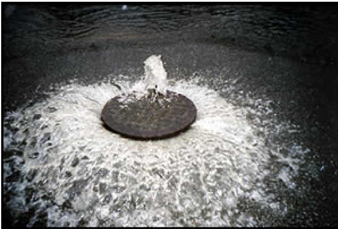
Figure 5.40: Overflowing Sanitary Sewer A manhole cover blown off by a June 2006 sanitary sewer overflow in Rhode Island. Source: U.S. Environmental Protection Agency 47 via Wikimedia Commons
