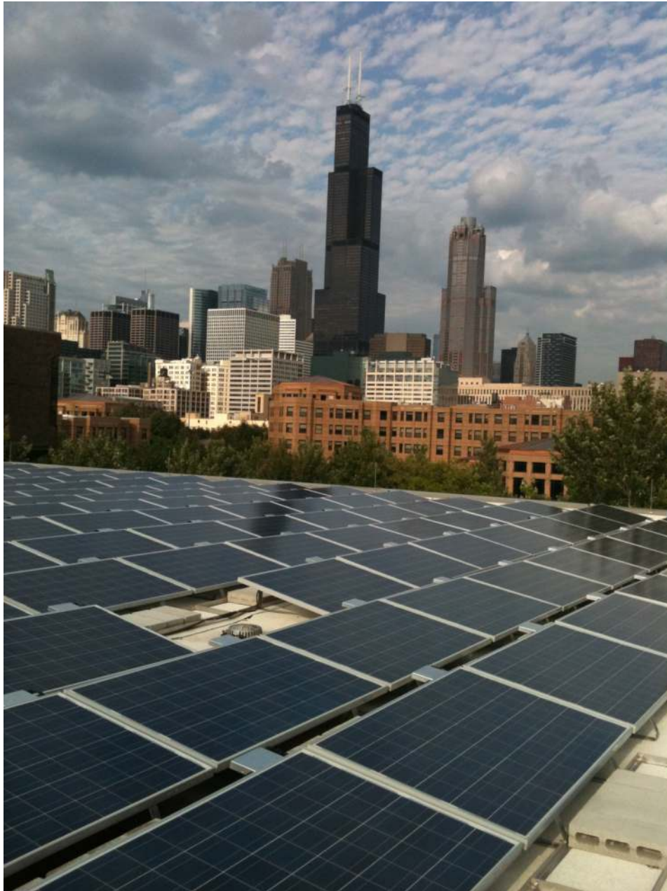
Figure 8.17: Rooftop Solar Installations Rooftop solar installation on Douglas Hall at the University of Illinois at Chicago has no effect on land resources, while producing electricity with zero emissions. Source: Office of Sustainability, UIC 47
