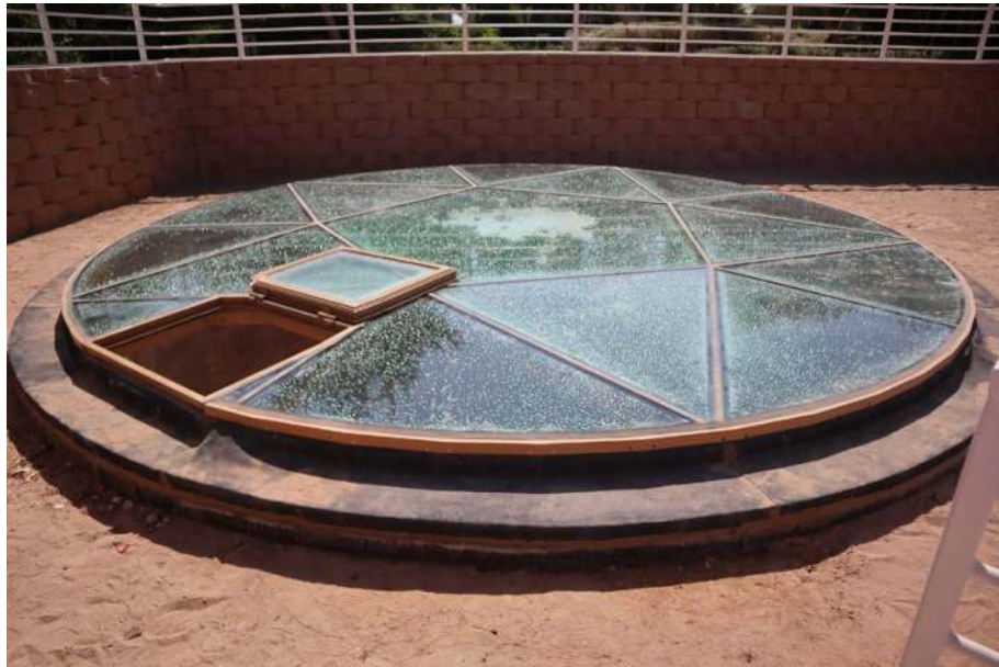
Figure 15: The glass cover over the thugba in Unit 4. (DCT Abu Dhabi, 2022)
