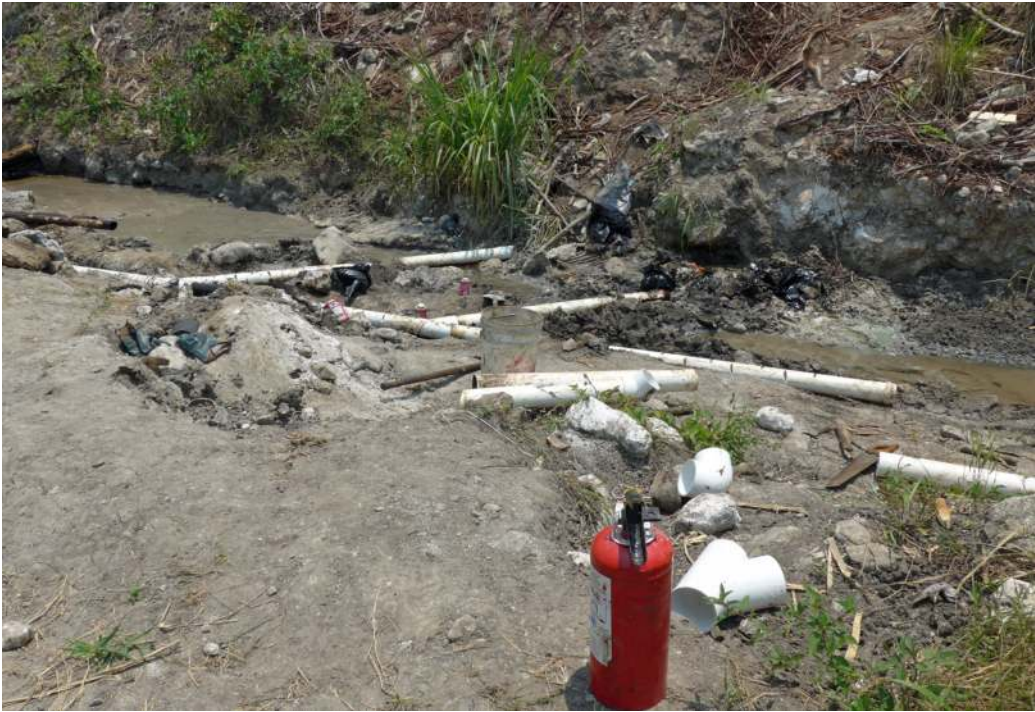
Figure 4.1. A month-old seepage within the river, which awaits repairs, Papantla, Mexico, 2017 © Svenja Schöneich.
