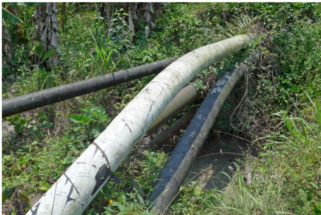
Figure 4.4. Pipelines protruding in a field in Emiliano Zapata, Papantla, Mexico, 2017 © Svenja Schöneich.
